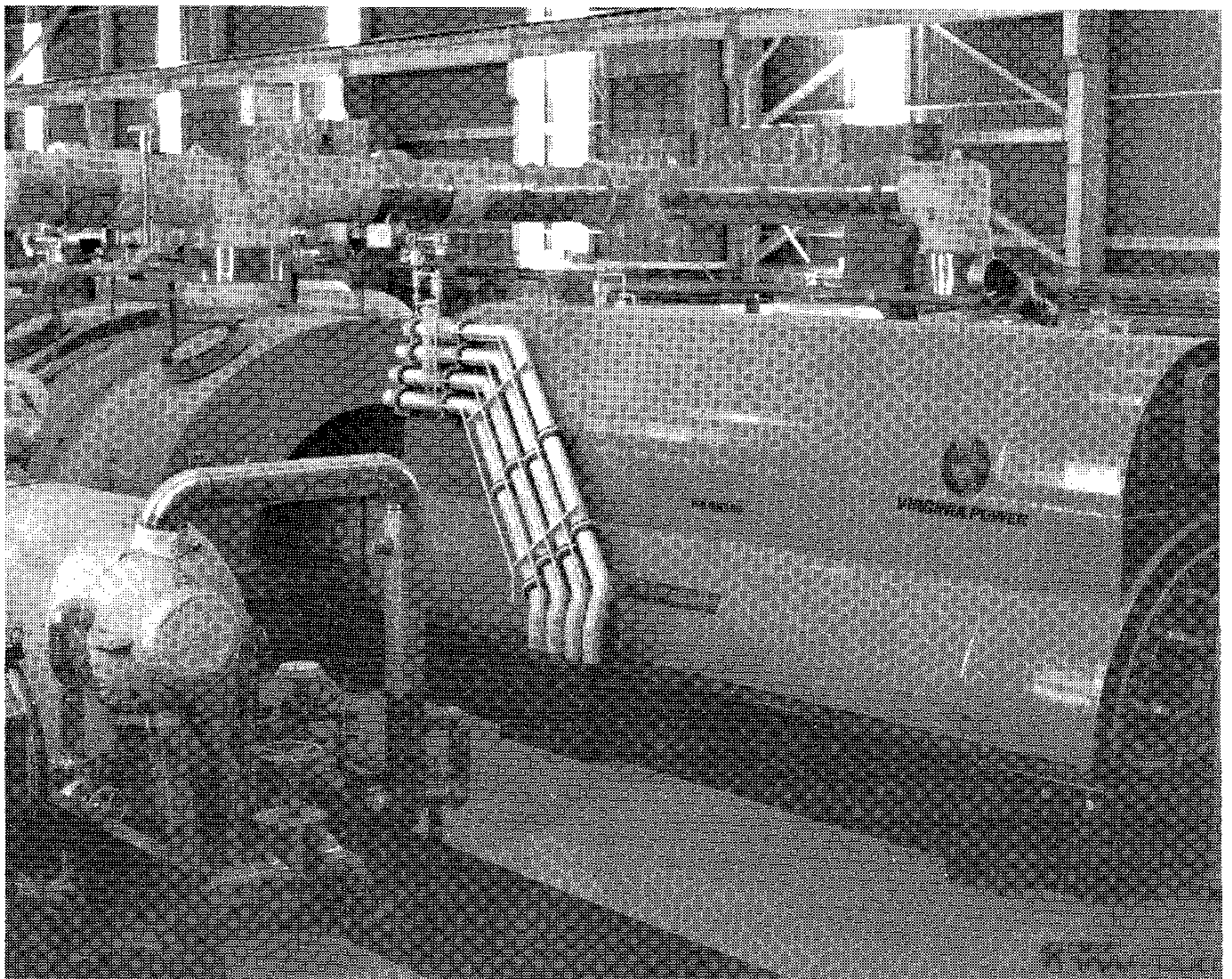
Fig. 19. The main turbine
